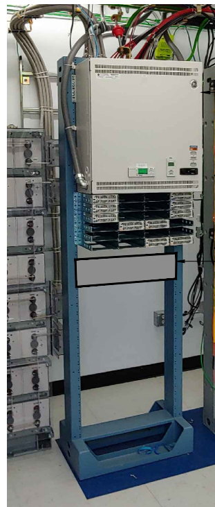
EXISTING PDF RACK
