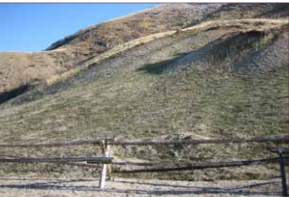
Image above (top): Before restoration. Image at right: Restoration activities. Image above (bottom): After restoration.
